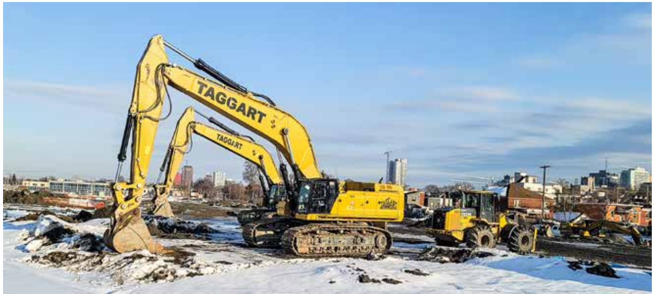
Left: Mosaïq phase 2 on the south side of Gladstone at Rochester. Above: Gladstone Village near LRT Line 2. CHARLES AXBEN-MARCHAND/THE BUZZ
