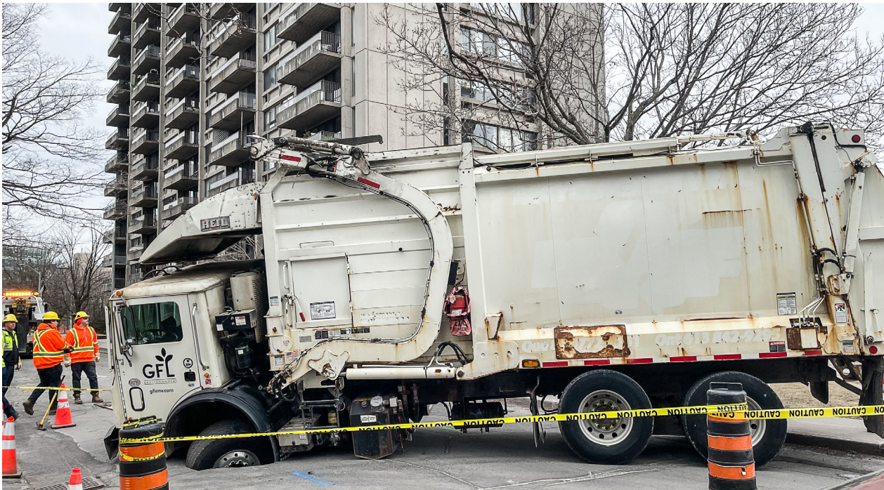
One of the classic signs of spring is the pothole, but this one on Cooper was a doozy! BUZZ reader Nancy Walking captured this scene on March 26 in front of her building. The front left wheel of a garbage truck was captured by a large hole in the street, completely blocking all traffic. NANCY WALKING/THE BUZZ
