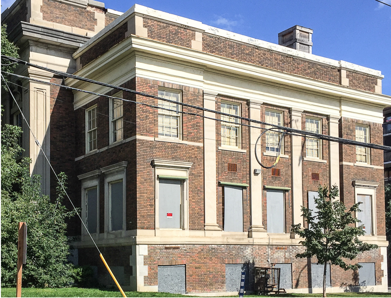
The 1922 section of 330 Gilmour (seen here from O'Connor Street). Many windows are boarded up.
