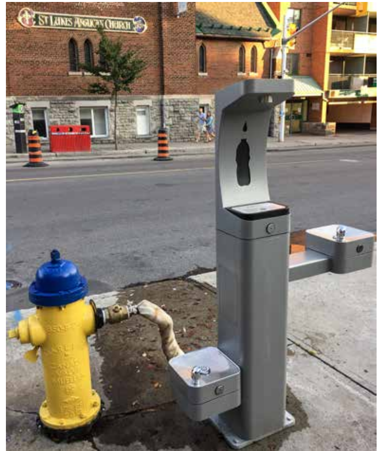
The City of Ottawa unveiled its first hydrant drinking water fountain in August, with a two-week trial run at Somerset Street West and Empress. It’s now looking for feedback, and may install more fountains next summer to provide refreshment during heat waves. ALAYNE MCGREGOR/THE BUZZ
