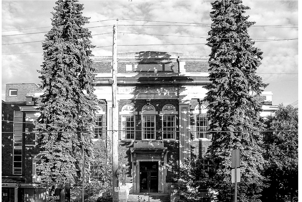
The former Ottawa Board of Education headquarters on Gilmour Street, now owned by Ashcroft Homes, has been vacant for over 20 years. Serious wall and foundation settlement is now occurring. It has recently been boarded up in an effort to prevent further water penetration.
