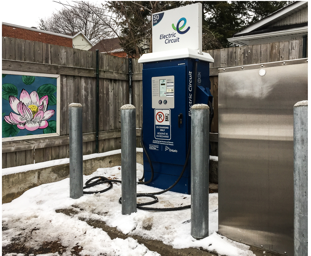
This new EV charging station for electric cars is located in the parking lot at Somerset West and Cambridge Streets. The City of Ottawa is now looking for more locations for these stations, in areas with more rental housing, higher population density, lower income levels, and less frequent public transit. You can suggest a location on the city's online map. Beside the station is a community mural installed in 2020 by The Door Youth Centre, with the theme "Flowers of Asia." ALAYNE MCGREGOR/THE BUZZ
